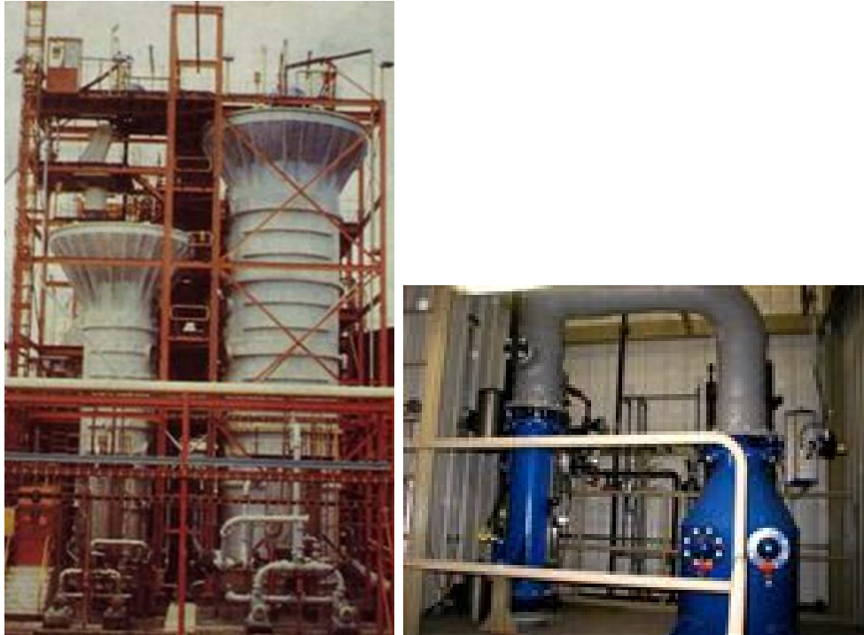
Figure 12 NIMCIX Equipment 5 and Higgins Loop System 6
