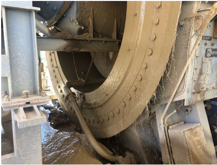
FIG 6 – Excessive Ball mill feed spillage.
