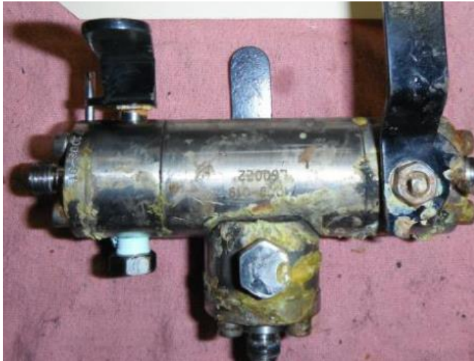
Ball Valve Body Leakage
