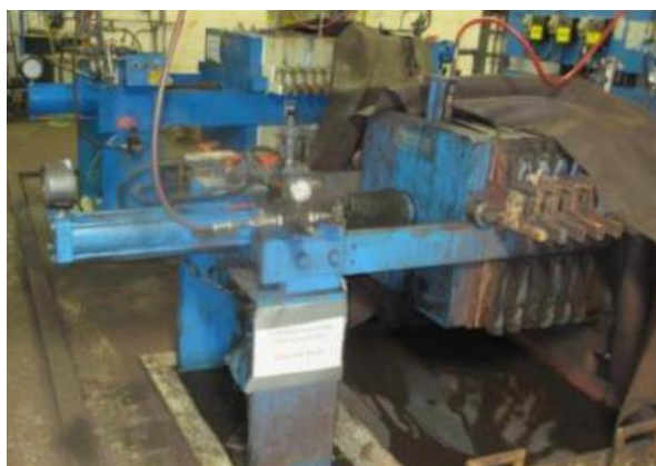
Figure 25: Demonstration Plant Filter
