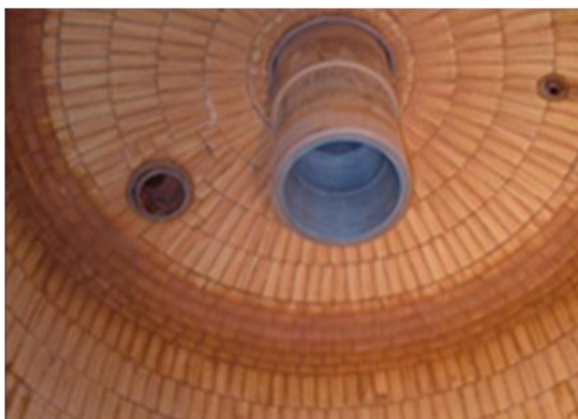
Figure 10: Upgrade Autoclave Flash Tanks Internals
