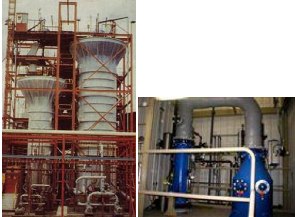
Figure 12 NIMCIX Equipment 5 and Higgins Loop System 6
